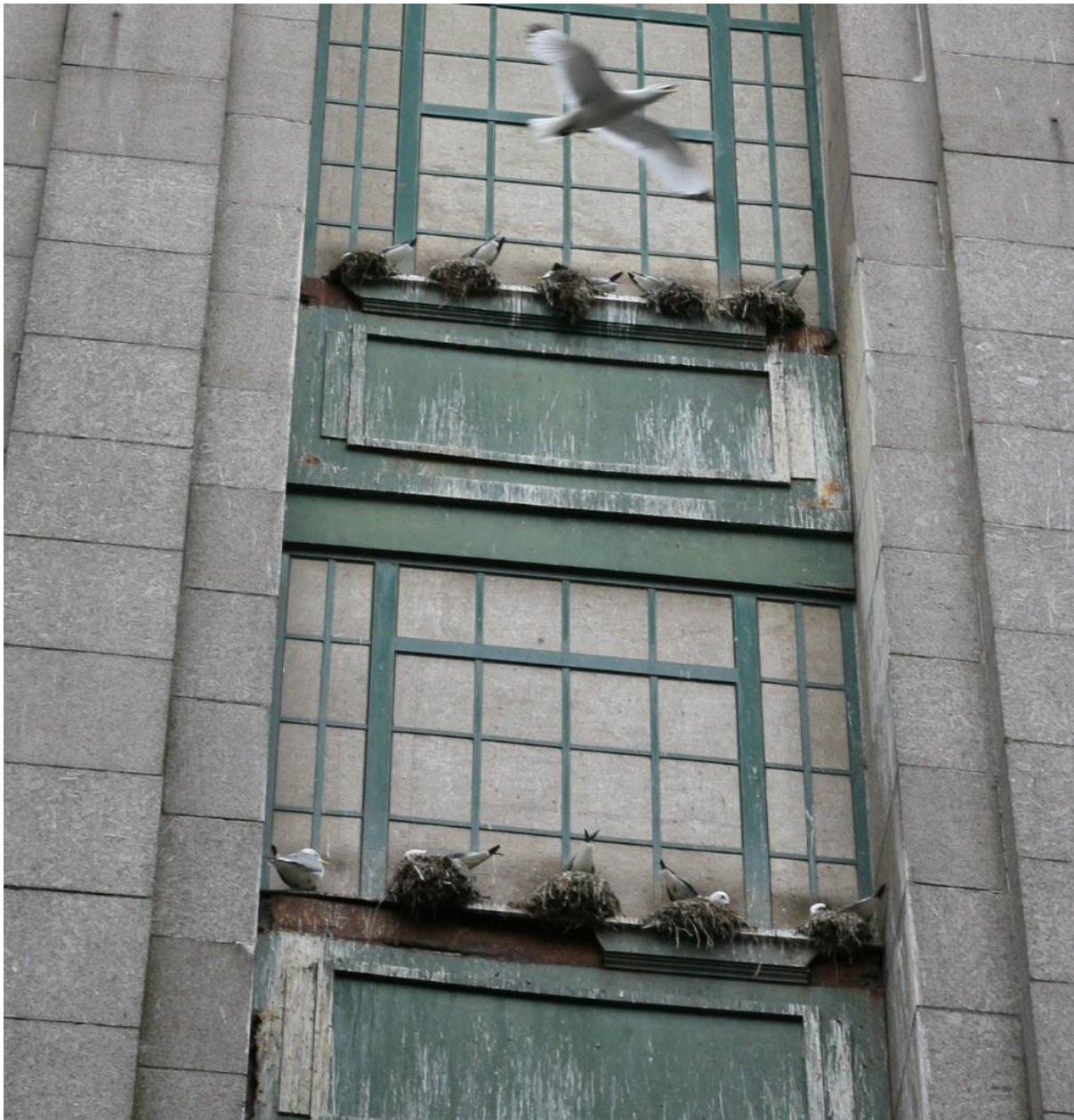
Photo 4.1.1. Some of the narrowest ledges used by kittiwakes are on the Tyne Bridge where chipboard covers have been placed over the windows of the bridge abutment towers below the road level.
